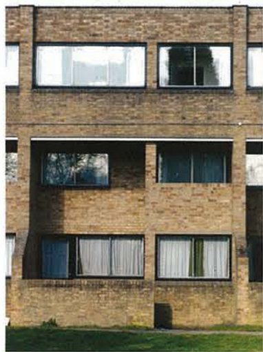
1 Courtyard elevation of the Wolfson Flats at Churchill College after its rehabilitation. 2 Before renovation.
